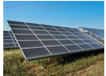
Examined PV power plant in Italy
