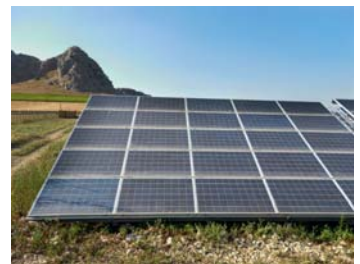
Examined PV power plant in Italy
