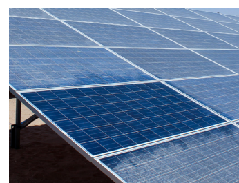
A cleaned PV module alongside soiled modules
