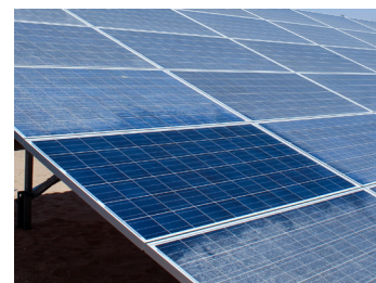
A cleaned PV module alongside soiled modules
