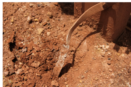
Figure 1: Ground electrode affected by salt corrosion
